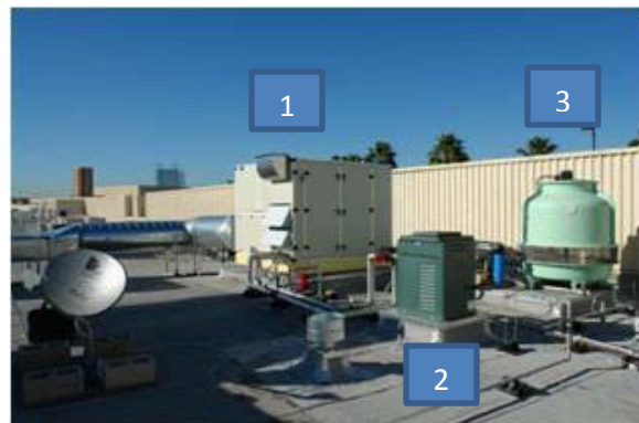
Figure 2: Major components and packaging of the AILR LDAC (Photograph shows packaged HMXs, water heater and cooling tower)
